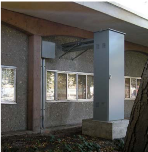
Cabinet outside of Chabot College Building 200
