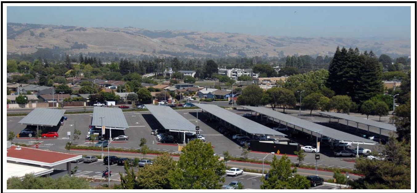
Lot G with Photovoltaic
