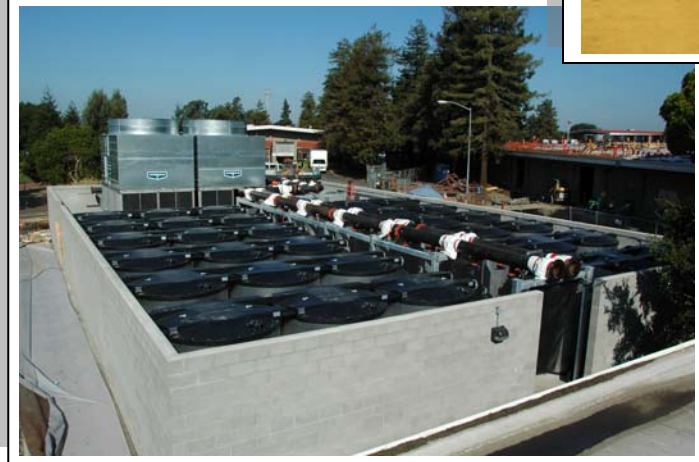
Ice Storage Plant
