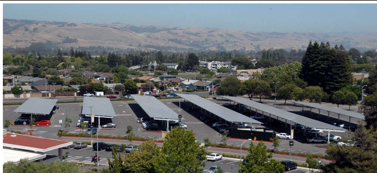
Lot G with Photovoltaic
